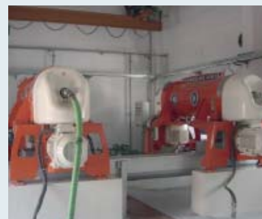
Impianto municipale trattamento acque reflue Municipal waste water treatment plant - Station d'épuration des eaux usées ménagères
